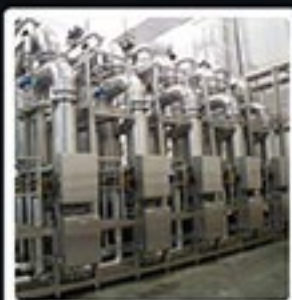
ULTRAFILTRATION PLANT FOR POLYMER RECOVERY FROM ORGANIC SOLVENT SOLUTION
